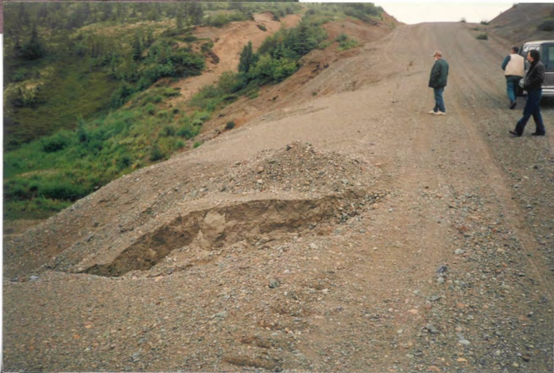
Road from Iliamna - erosion apparent at culvert
