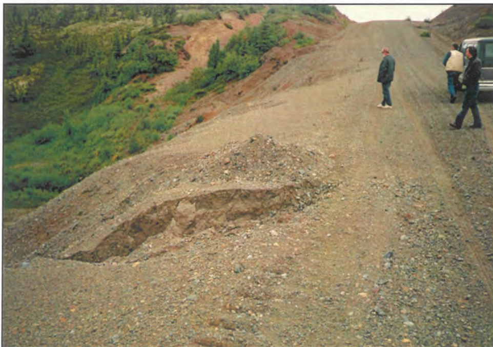
Photo 10: Typical view of erosion along the Iliamna-Nondalton Road. Photo probably taken in 1995.
