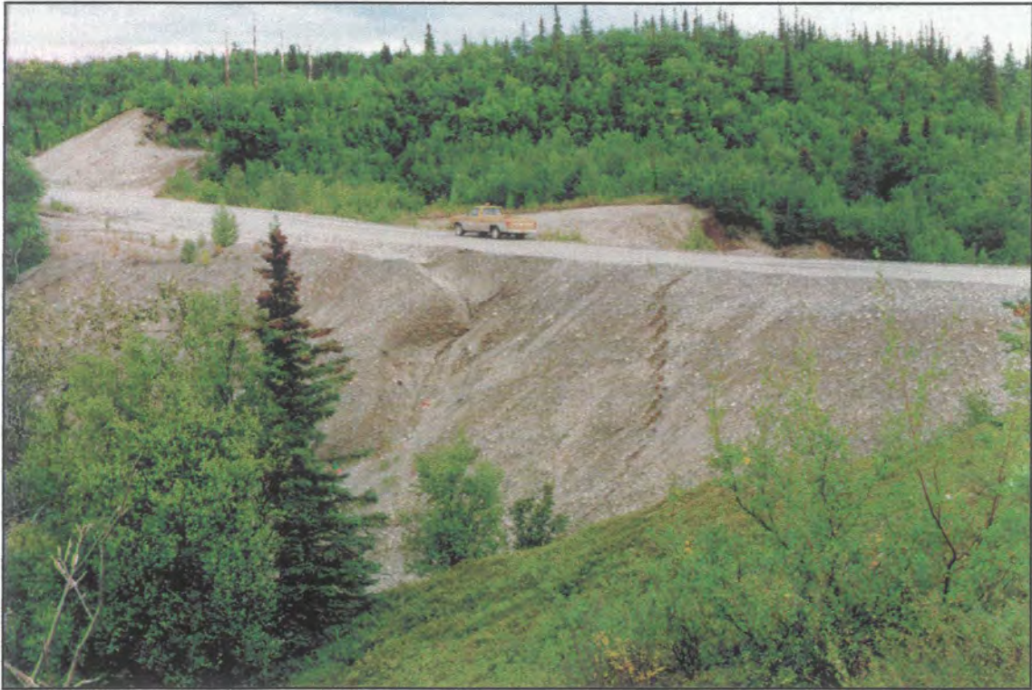
Photo 13: Eroded road embankment at Lover's Creek. 8-24-99.
