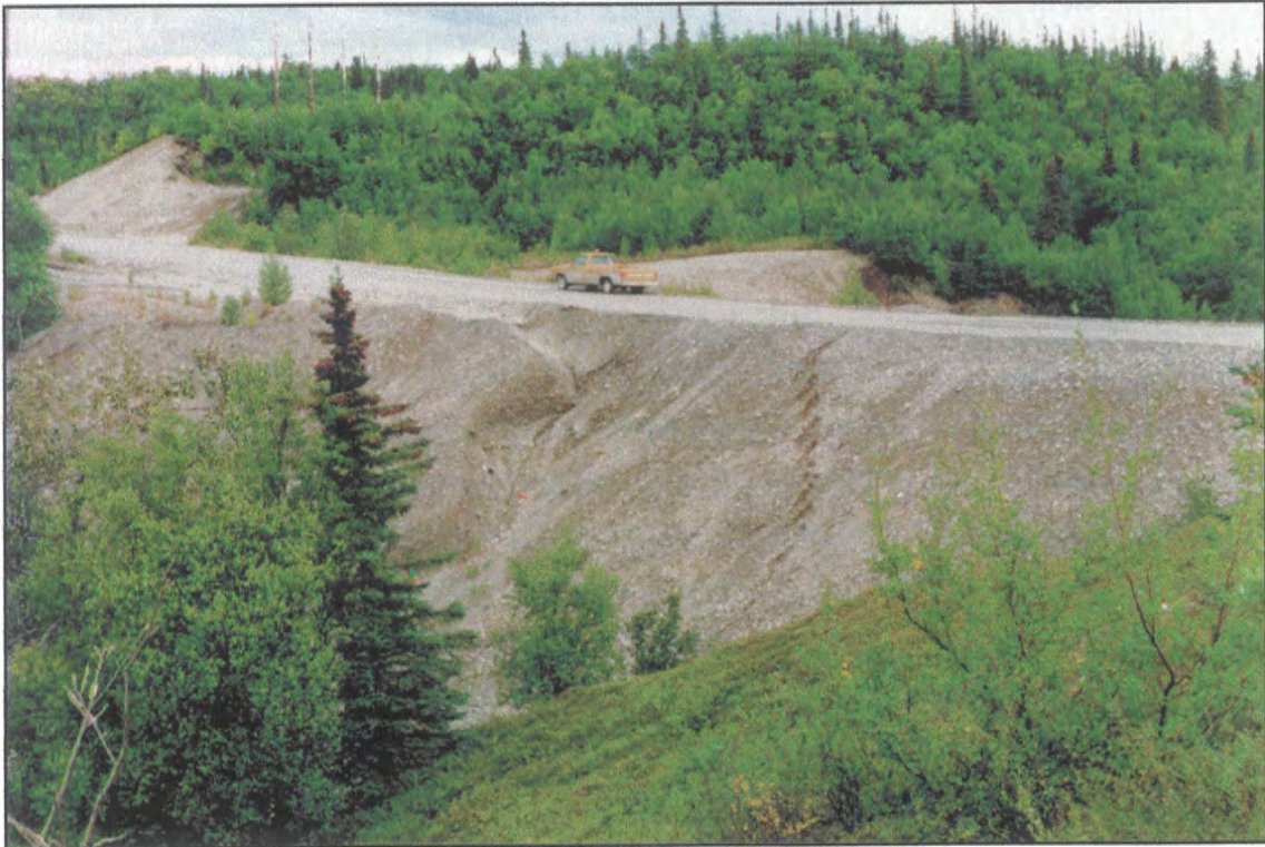
Photo 13: Eroded road embankment at Lover's Creek. 8-24-99.
