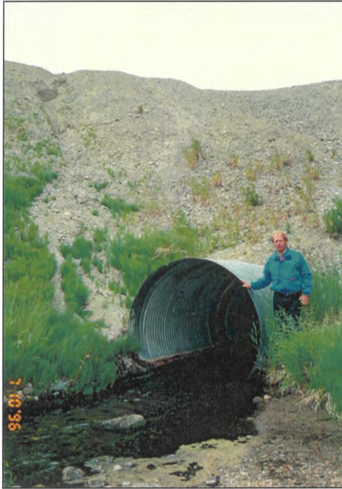
Photo 9: Large culvert and eroded bank along the Iliamna-Nondalton Road. 7-10-96
