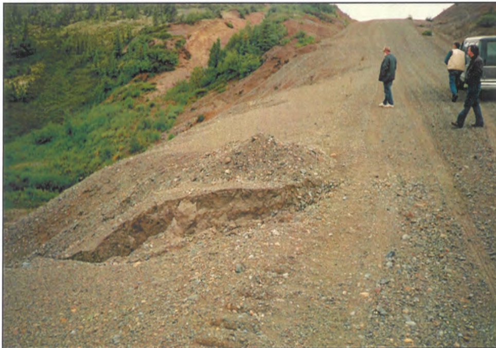
Photo 10: Typical view of erosion along the Iliamna-Nondalton Road. Photo probably taken in 1995.
